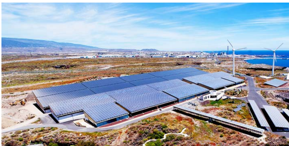
Figure 8.4.1. Photovoltaic plant located in the Institute of Technology and Renewable Energies (ITER) in the south of Tenerife
