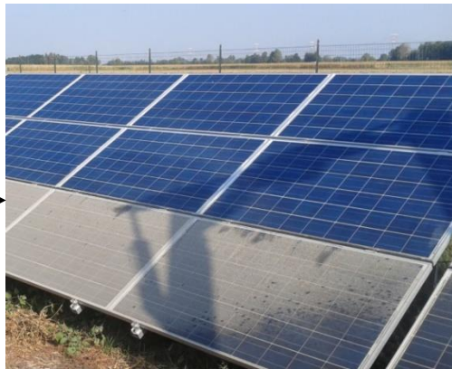
Soiled PV panel →
